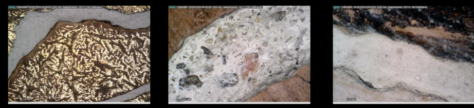
Upper horizontal crack Middle horizontal crack Lower horizontal crack
